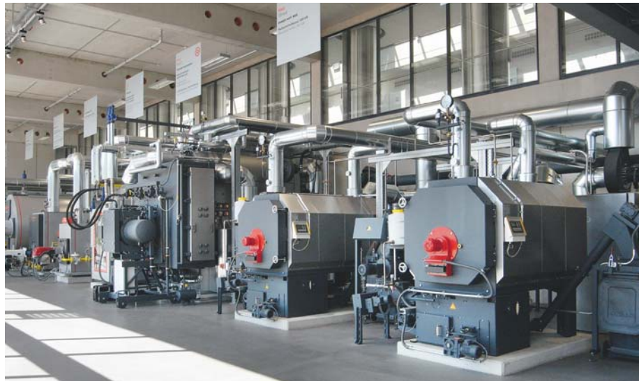
The energy centre was also designed for the generation of heat and power from sustainable fuels.
